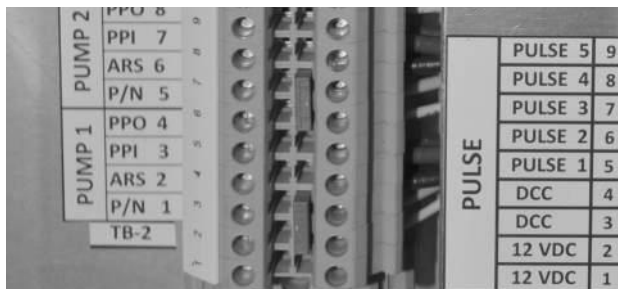
Figure 19. Pump 1 Connections on TB-2 - close-up
