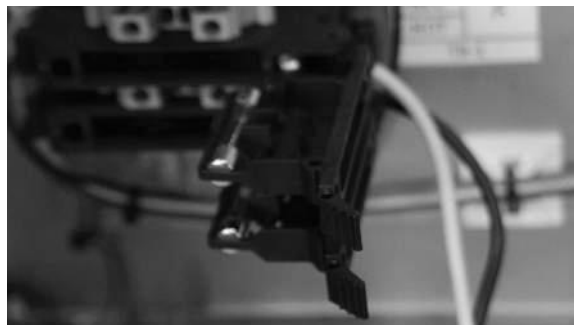
Figure 14. Fuse Handle in the Out Position
